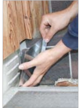
Adhesion of stainless steel to concrete bases
